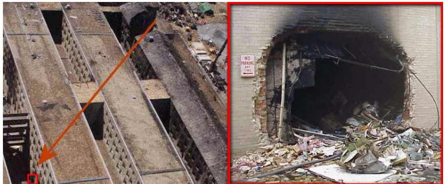
Penetration details of the Pentagon; 6 capital walls were penetrated and the final punch-out hole.
